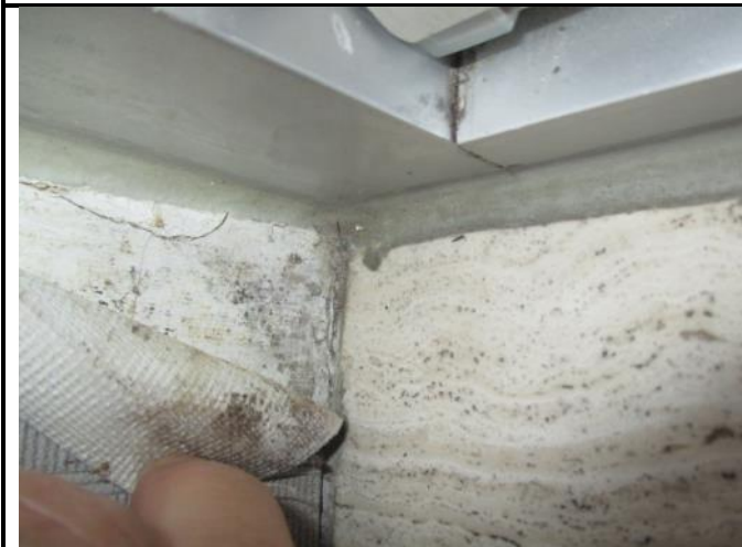
Photo 17: Lobby – example of minor mold growth behind lower edge of wallpaper at windowsill
