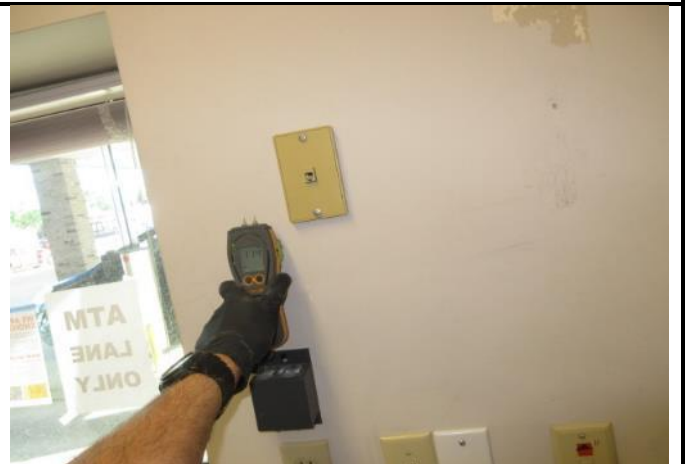
Photo 6: Tested location of drive-thru teller office north wall measured dry (114 REL)
