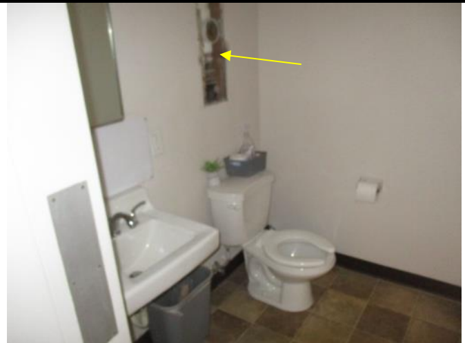
Photo 8: South restroom – reported plumbing leak repair location
