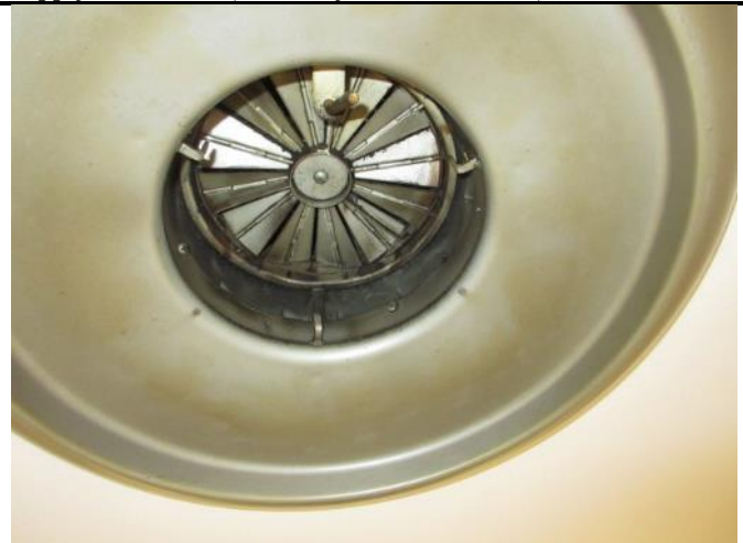
Photo 34: HVAC – louvres for supply vent diffuser outside south restroom are closed
