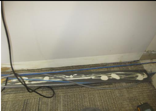
Photo 7: Exposed drive-thru teller office north wall lower drywall appears generally clean
