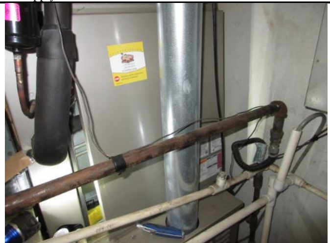
Photo 30: Southwest AHU – overview
