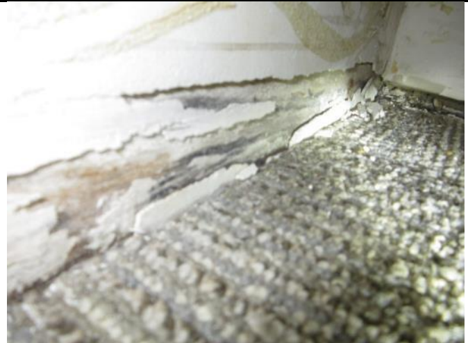
Photo 10: Example of suspect mold on lower plaster and sill plate below drive-thru teller office west return air inlet
