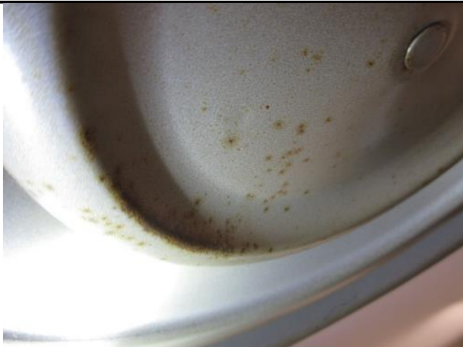
Photo 33: HVAC – example of visible mold on supply vent diffuser outside south restroom
