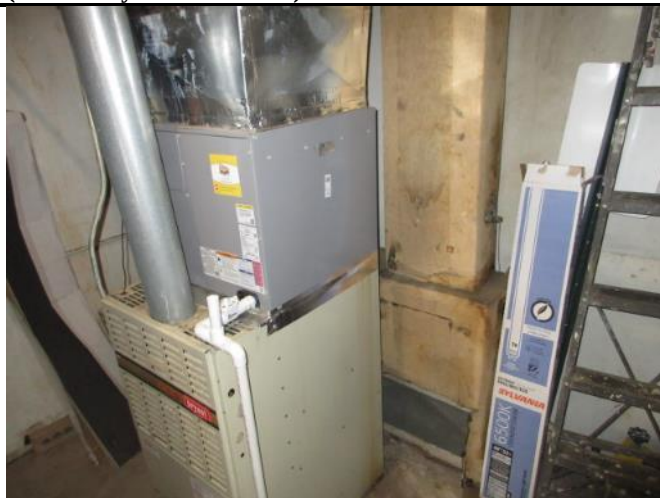
Photo 23: North HVAC AHU – overview
