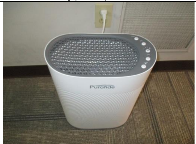
Photo 18: Drive-thru teller office – view of HEPA air filter
