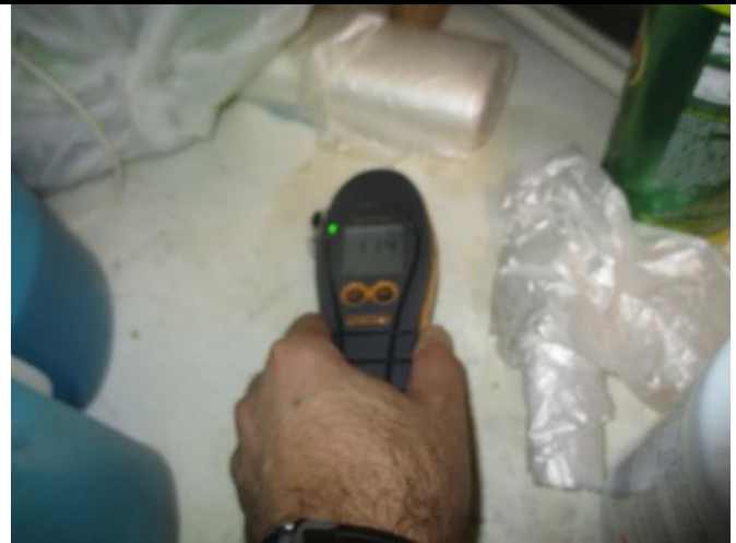
Photo 14: Break room – tested location of affected sink cabinet base shelf measured dry (114 REL)
