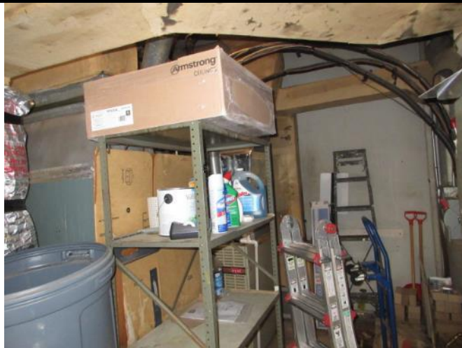
Photo 19: HVAC closet – overview
