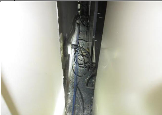
Photo 5: Example of dust and construction debris behind drive-thru teller counter
