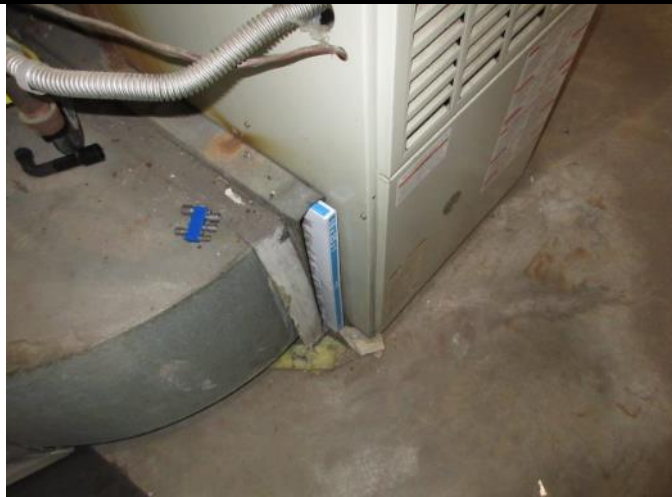
Photo 25: North HVAC AHU – air filter is improperly fit – no cover on filter slot
