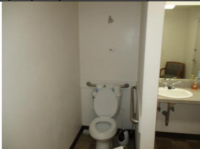
Photo 11: North restroom – example of damaged south wall plaster & button board wall above toilet
