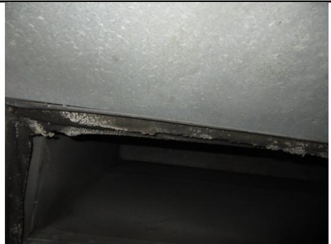
Photo 28: Southeast HVAC AHU – example of visible mold on supply trunk boot
