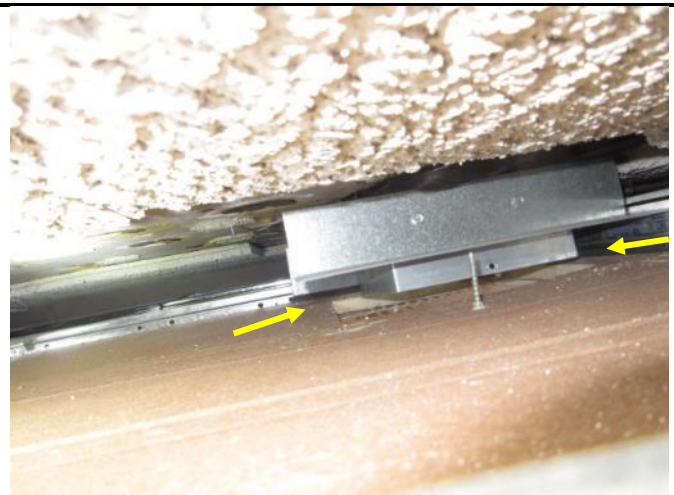
Photo 36: HVAC – example of gap between break room supply vent boot and lay-in ceiling tiles
