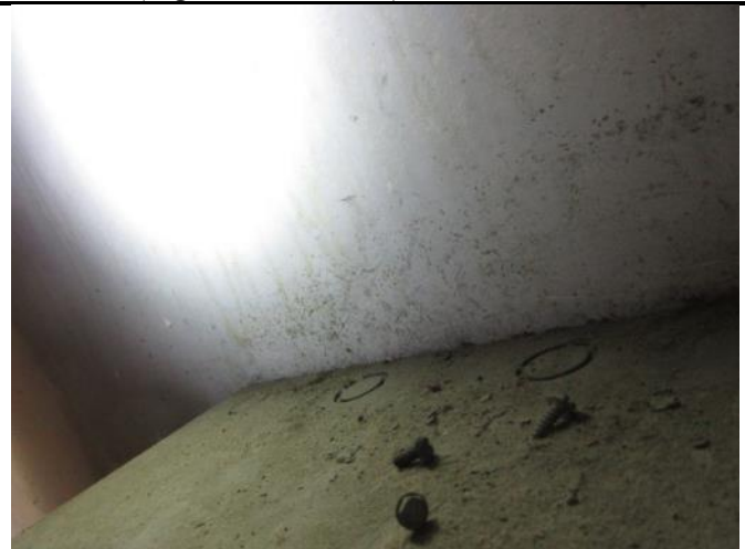
Photo 22: HVAC closet – example of visible mold on plaster wall
