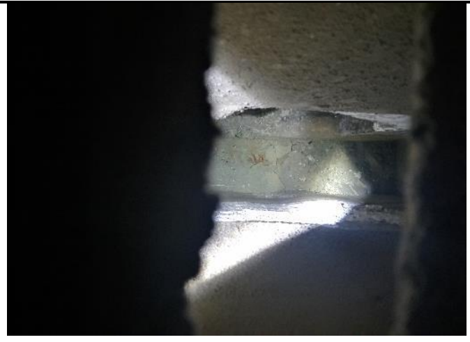
Photo 16: Example of standing water in lobby HVAC return air duct
