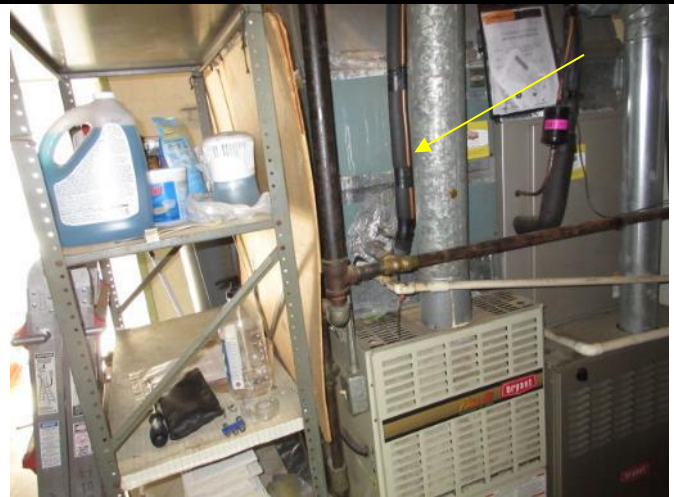
Photo 26: Southeast HVAC AHU – overview
