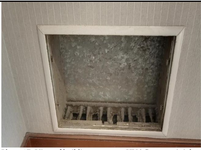
Photo 17: View of building rear entry HVAC return air inlet
