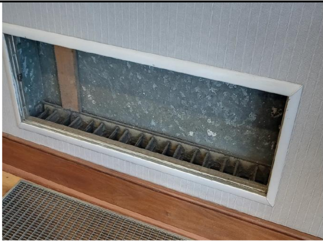
Photo 15: View of lobby HVAC return air inlet
