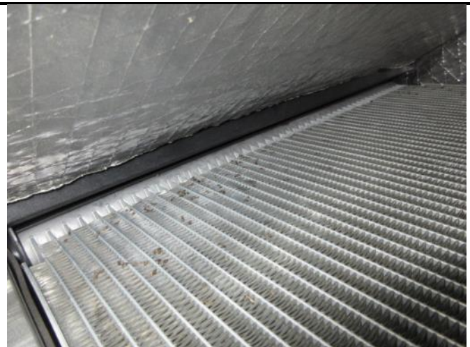
Photo 24: North HVAC AHU – example of minor visible mold on chill coils
