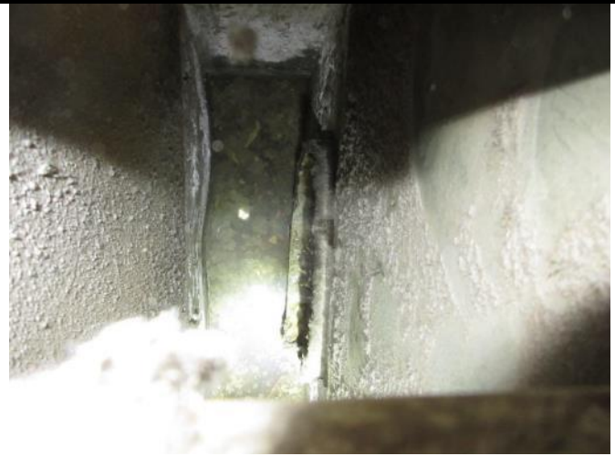
Photo 14: Example of standing water in drive-thru teller office HVAC west return air duct
