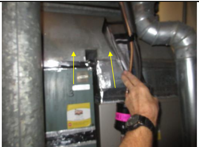
Photo 29: Southwest AHU – the AHU appears to service the same main supply trunk as the southeast AHU
