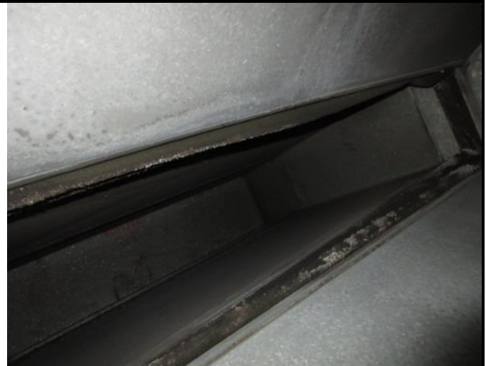
Photo 32: Southwest AHU – example of visible mold on main supply trunk boot (shared by southeast AHU)
