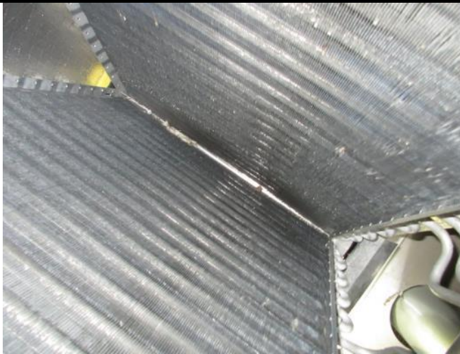
Photo 31: Southwest AHU – example of minor suspect mold on chill coils
