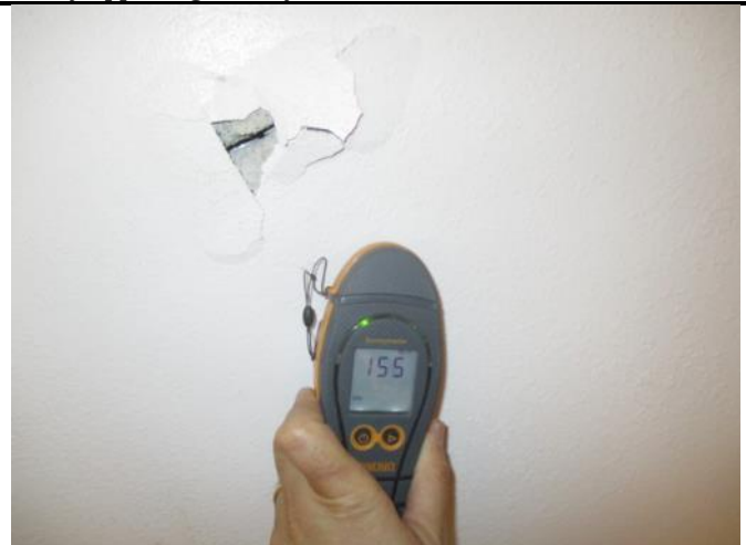
Photo 12: North restroom – tested location of damaged plaster & button board wall measured dry (155 REL)
