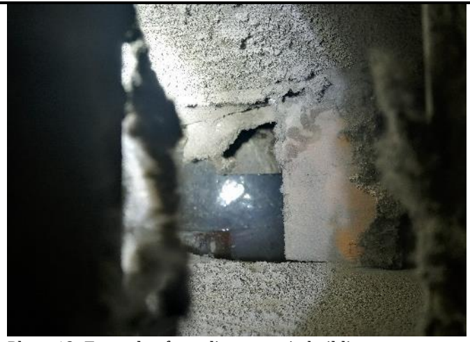
Photo 18: Example of standing water in building rear entry HVAC return air duct
