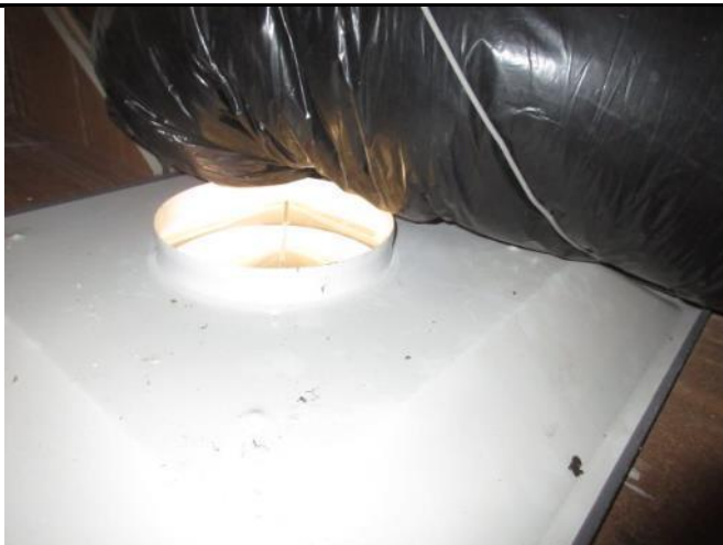
Photo 35: HVAC – example of detached supply flex duct at building rear entry
