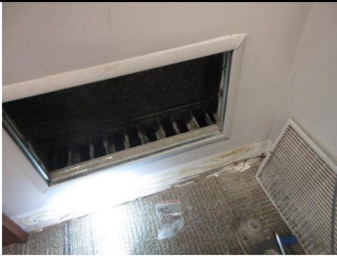
Photo 13: View of drive-thru teller office HVAC west return air inlet
