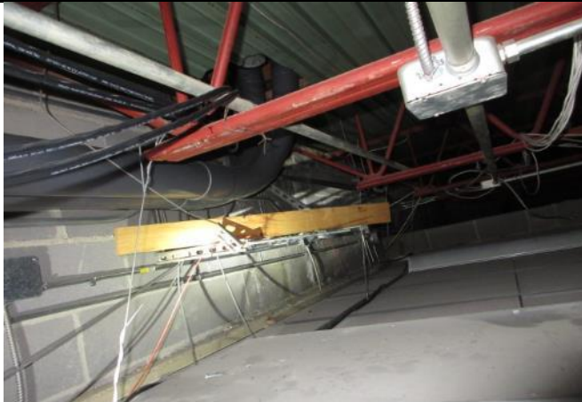
Photo 3: No access to the exterior overhang from within the building as viewed from the drive-thru teller office ceiling cavity
