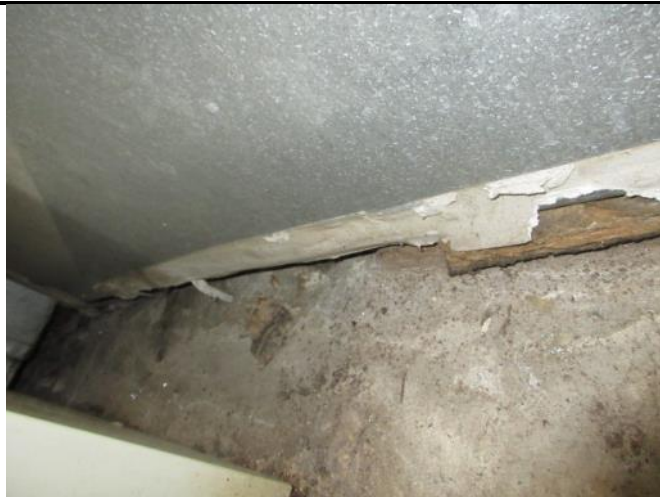
Photo 21: HVAC closet – example of white HVAC seam tape (40% Chrysotile asbestos)
