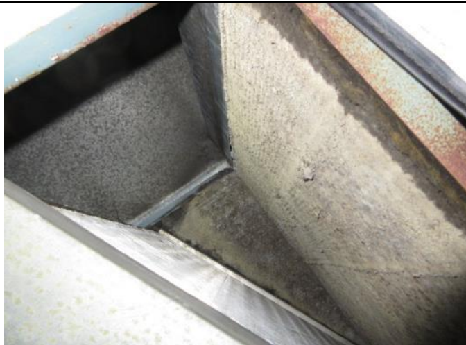
Photo 27: Southeast HVAC AHU – heavy accumulations of mold on AHU interior insulation
