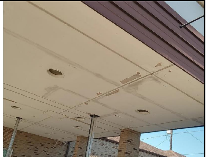
Photo 2: Example of apparent water damage on drive-thru overhang panels
